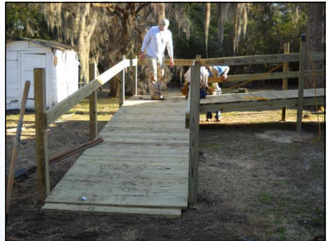
Dennis Corporation employee Thomas Inabinett and crew working on the construction of the handicap ramp.
