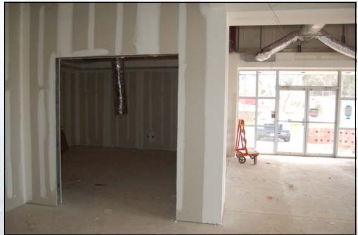
The Large Conference Room and Entry Way January 20, 2010
