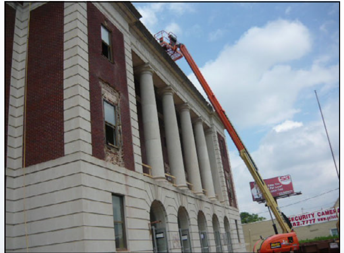
Dennis Corporation currently managing the construction of the Township Auditorium in Columbia.
