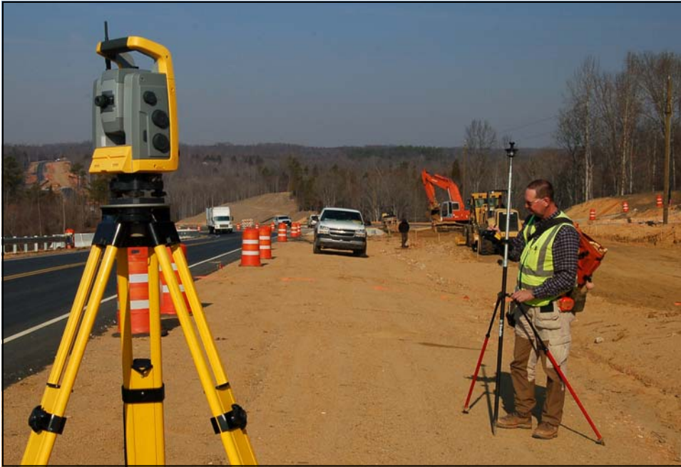
Dennis Corporation Survey Crew Chief, Jeff Gwin, utilizing the Robotic Trimble S6 on South Carolina Highway 5.
