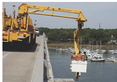
The photo above, taken by Christophe Mallet, shows workers inspecting the closed J.E. McTeer Bridge.
