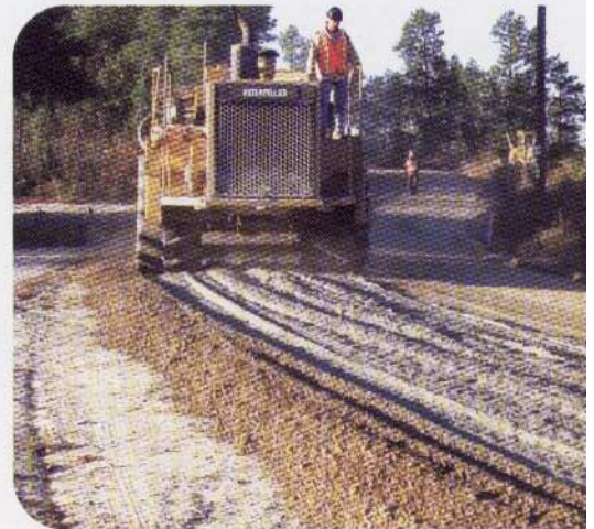
Mixing cement into the pulverized roadway to create a stabilized base. FDR with cement saved Fairfield County, S.C., taxpayers nearly $1.5 million.
